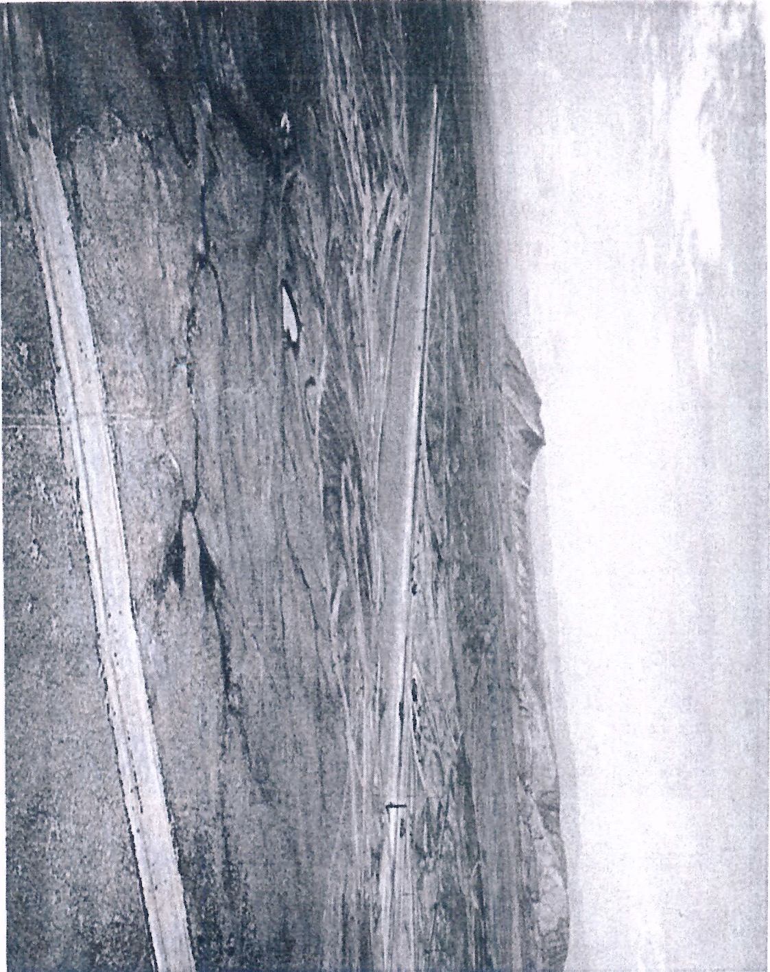
Morgan Lake Dam 80 % complete. Left part of photo (East) will become Morgan Lake. Small pond at lower left center is likely a stock tank constructed to catch rain water for stock watering. 9/14/61
